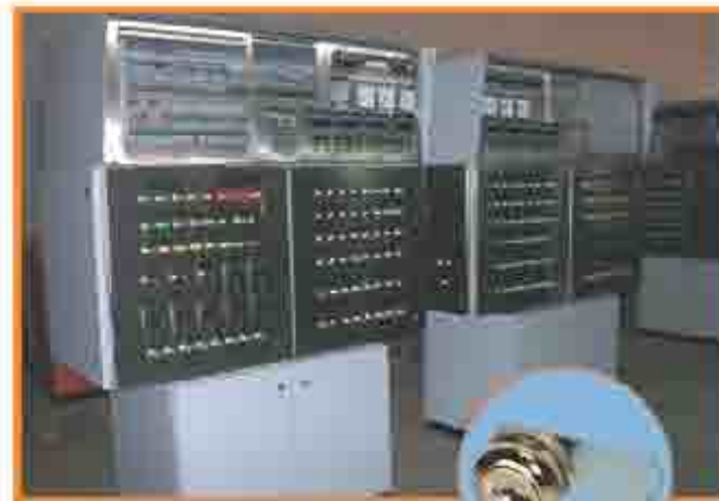
Control Station Special
